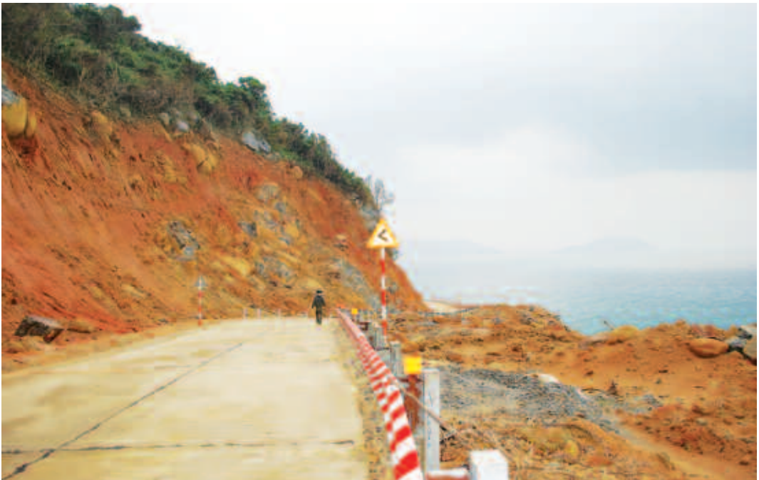
Fig.7. Roads create large gaps in the forest, which in some places are over 100 m wide. Photo: Ulrike Streicher.
