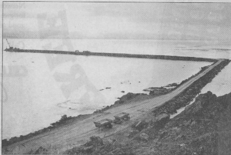
The west arm of the breakwater stretched 2,620 feet from Pillar Point. Together both arms used more than 800,000 tons of rock.
