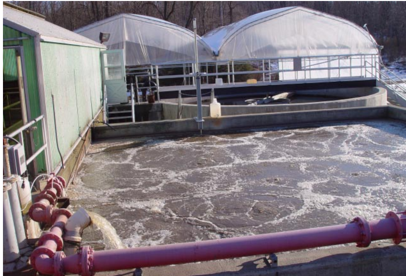
Figure 4: Waste Water Treatment Plant
