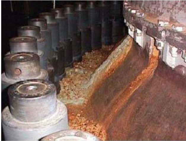
Red Rusty Boric Acid Deposits on Vessel Flange (12RFO)
