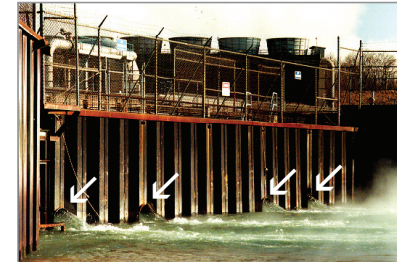
Water discharge area at the Palisades nuclear power plant on Lake Michigan. Note the flow from four big ejection outlets .
