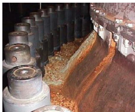
This is what inspectors ignored.
