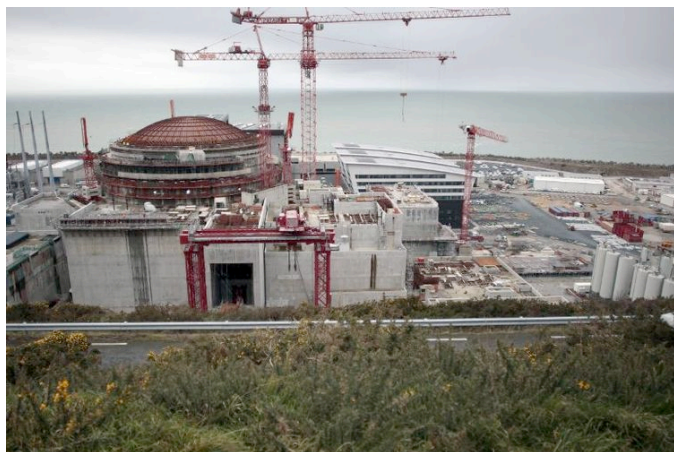
The once heavily touted EPR may never become anything more than a concrete white elephant. (Photo: Flamanville site in 2014.)
