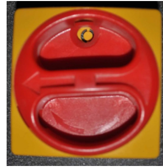
Control Box Power Switch
