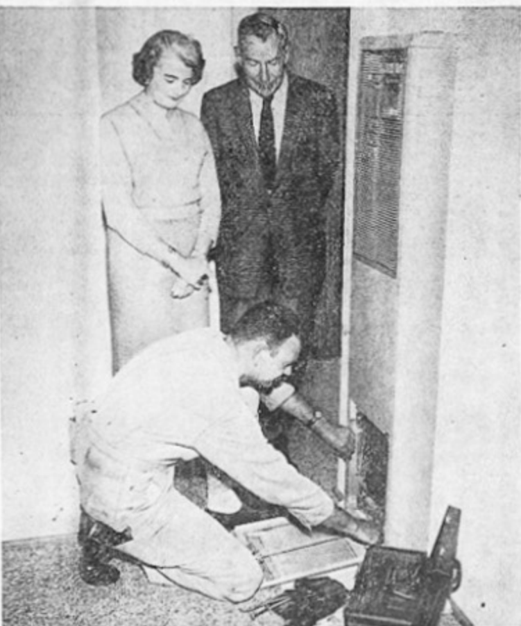
FIRST SERVICE — Serviceman R. D. Richards completes first natural gas installation in Cherry Valley at home of Mr. and Mrs. A. D. Bennett. Gas mains have been installed in the area just north of Beaumont to serve Cherry Valley.
