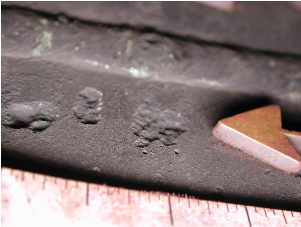
Detection and proper evaluation of internal corrosion is critical in pressure vessel inspection.
