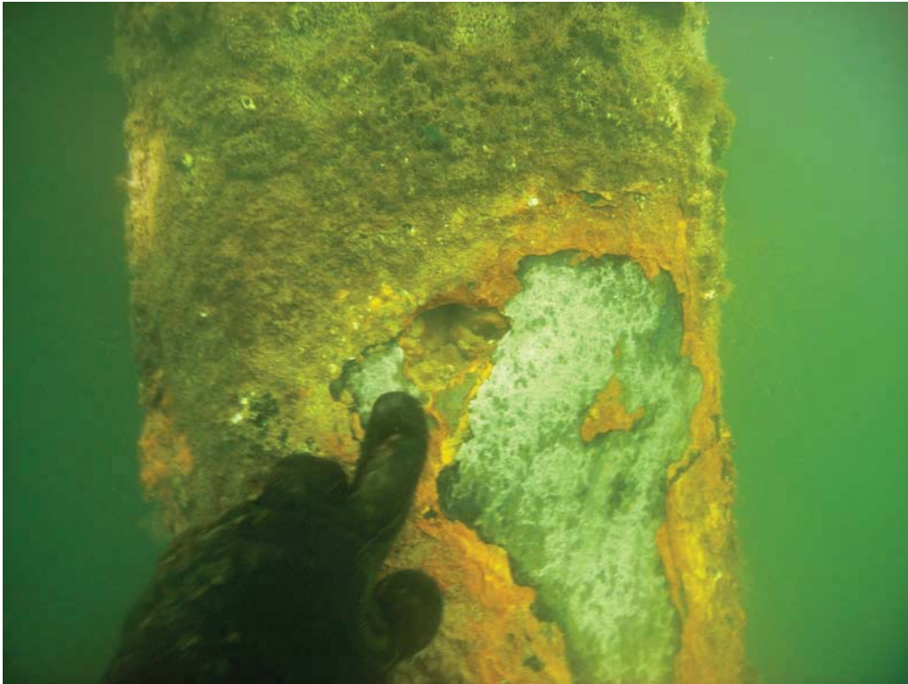
In some instances small holes in steel piles can be documented and repaired.
