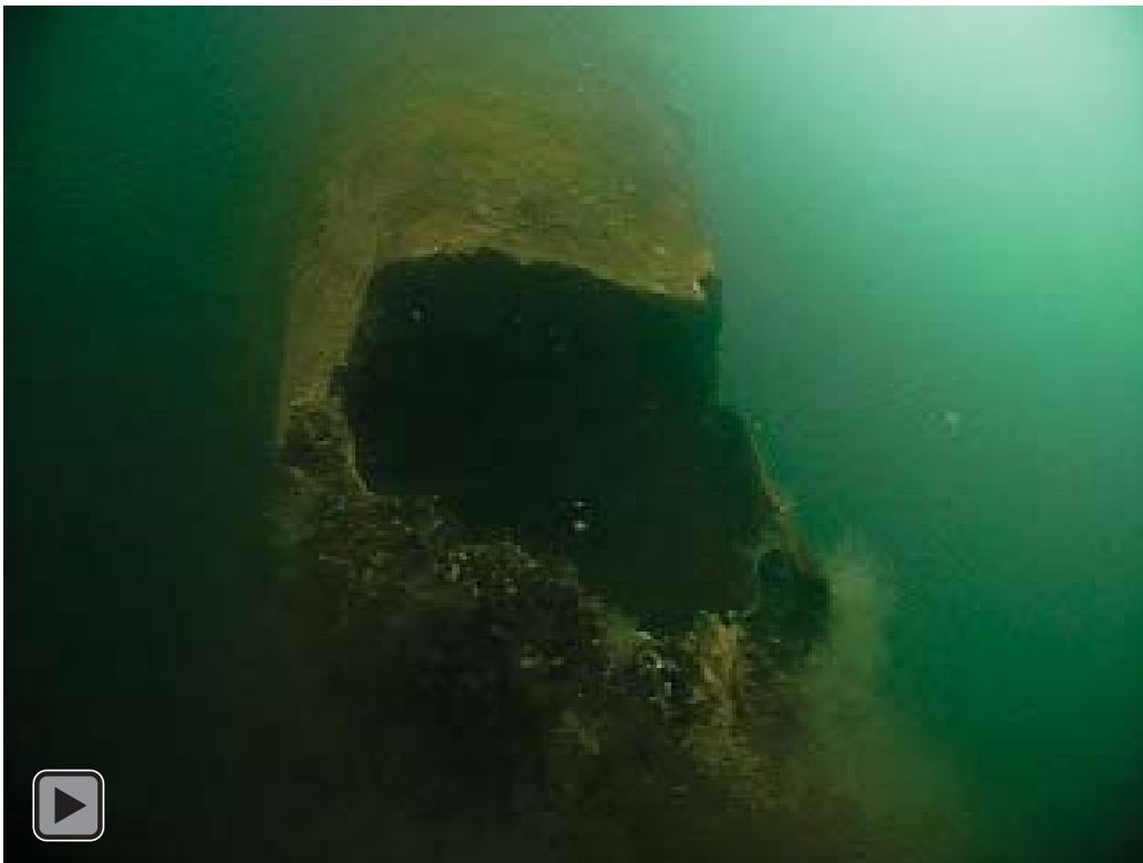
In some instances the structural integrity of the facility may need immediate action.
