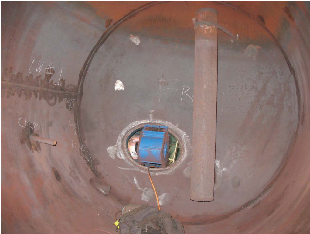
The initial task in Deaerator Inspection is cleaning all major pressure boundary welds.
