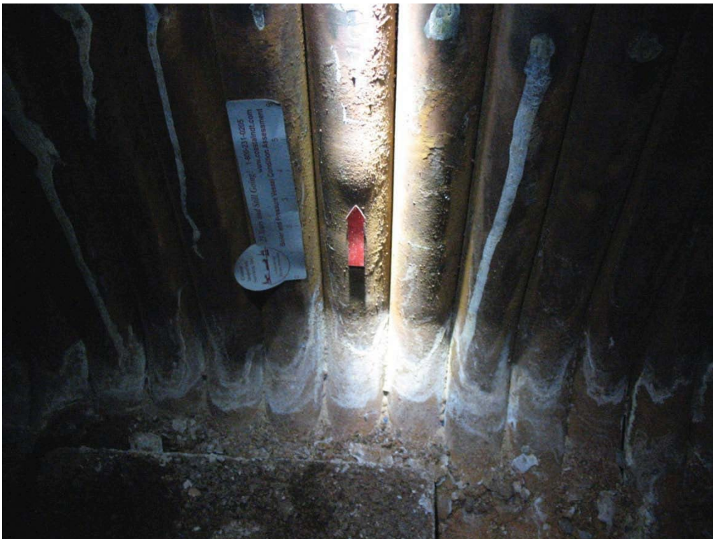
Blisters on furnace tubes often indicate loss of thermal transfer.
