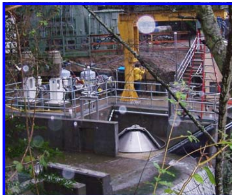
Above: Screen installed at shallow impoundment behind inflatable dam.
