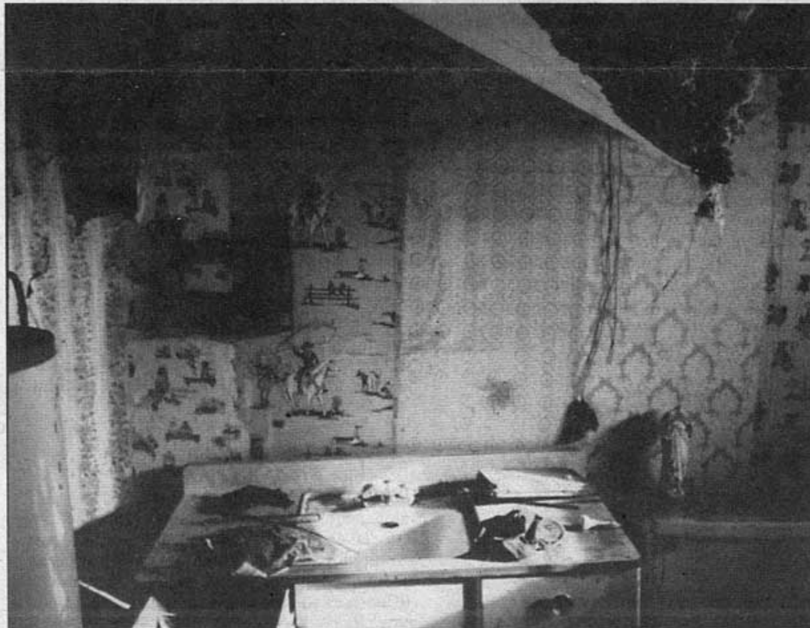
"Bathroom in a house in Model, eastern Colorado, February 11, 1994" is slowly losing its mismatched wallpaper; the shelves have been stripped clean; debris litters the sink; and a headless religious statue prays on the toilet tank.
