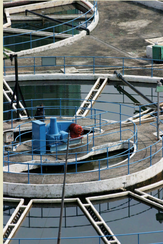
Reduce waste water treatment plants
