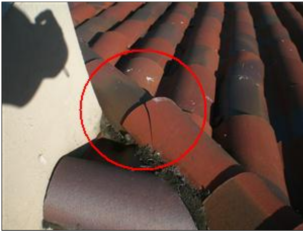
1.0 Picture 3 cracked tile
