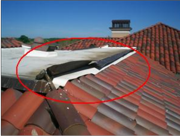
1.0 Picture 1 damaged flashing & missing tiles
