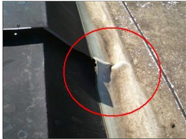
1.0 Picture 4 damaged roofing membrane
