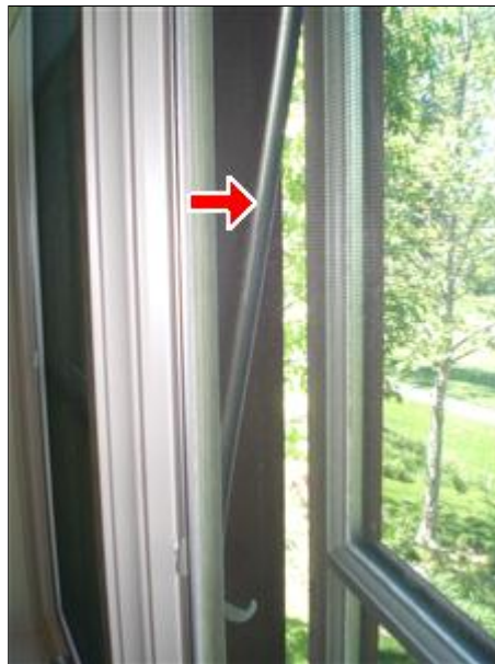
4.6 Picture 1 damaged seal
