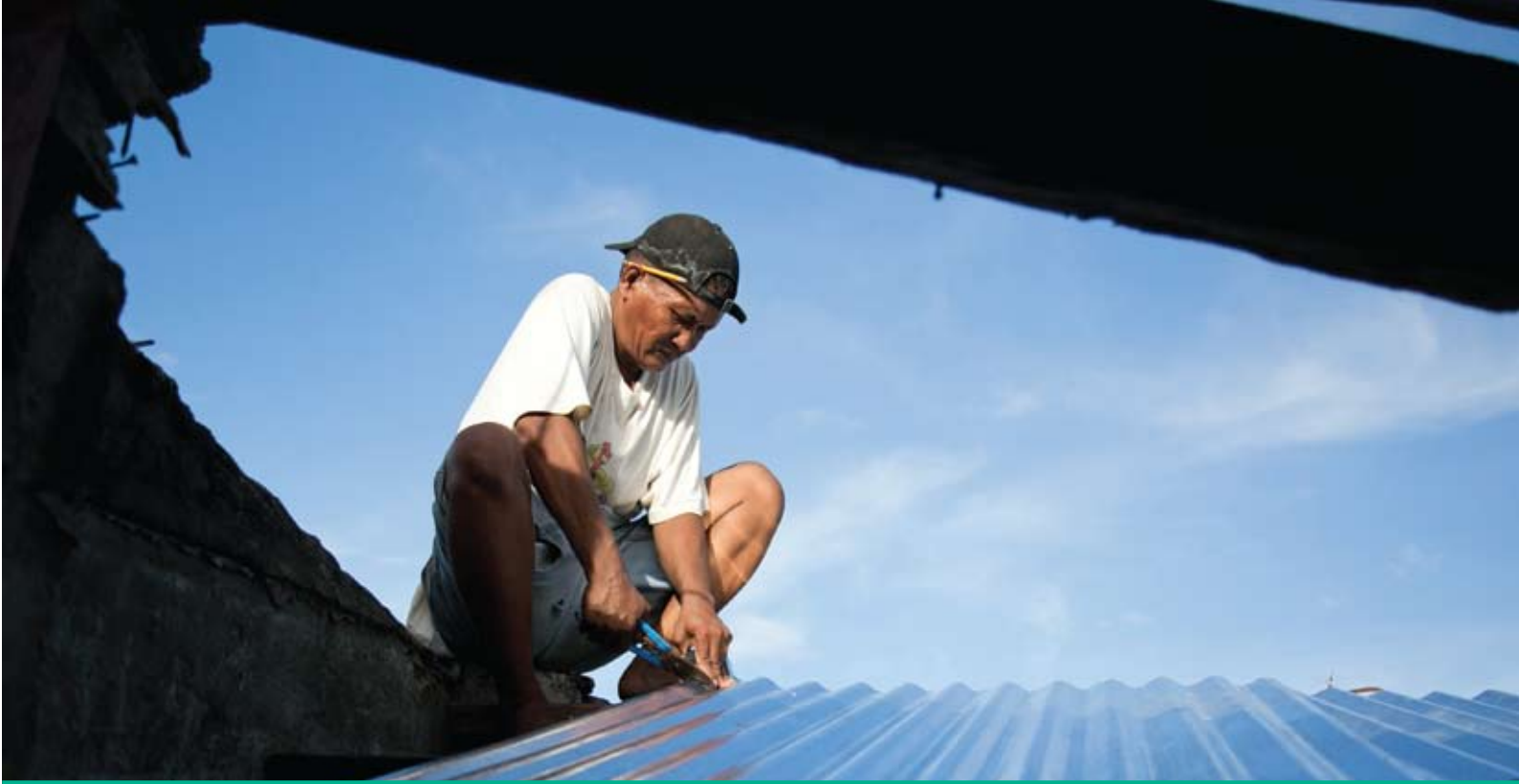
In all five locations, enforcement and public awareness of construction codes was low. Photo by Jennifer Hardy for CRS
