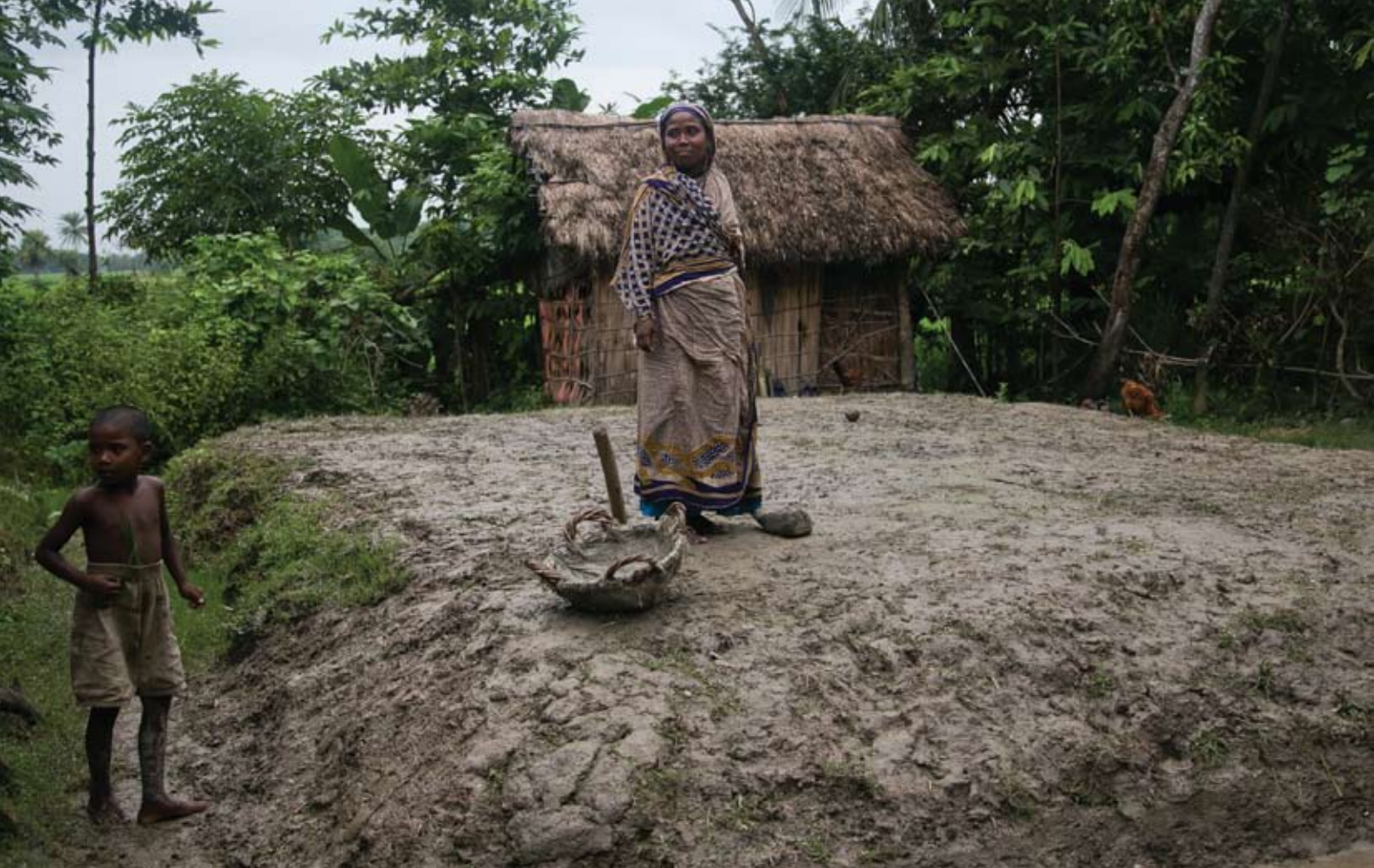
Rahima Begum works on building the raised plinth of her future home in southern Bangladesh. Photo by Jennifer Hardy for CRS
