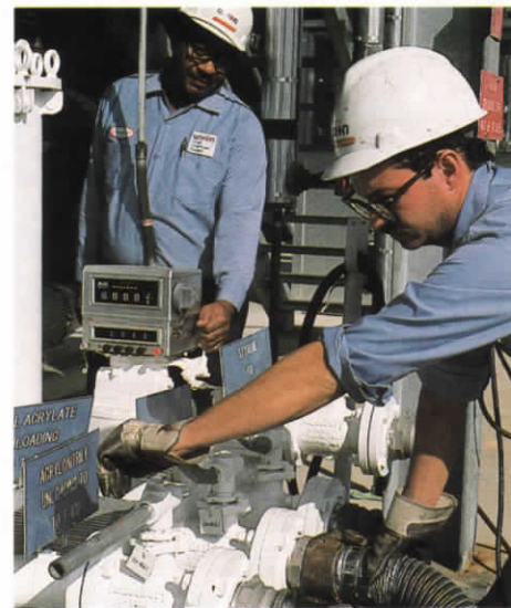
Leonard Witherspoon (left) and Butch Hammett prepare to transfer finished product into a rail tank car for shipping.
