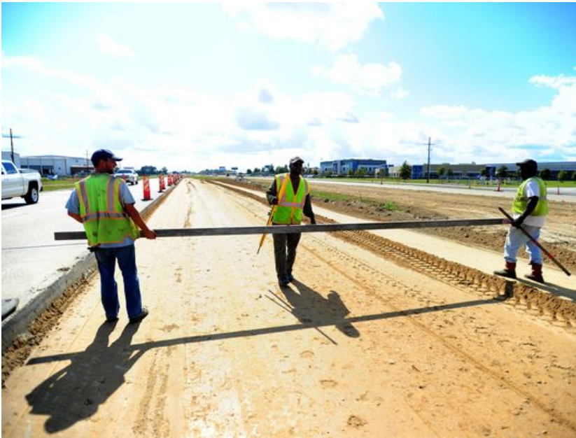
Highway workers continue road construction on U.S. Highway 90 in Broussard, LA, along the planned Interstate 49 corridor, Monday, Oct. 28, 2013. Paul Kieu, The Daily Advertiser (Photo: Paul Kieu, The Daily Advertiser)
