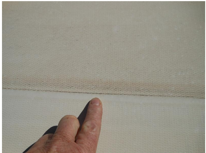
The top layer of polymer on this TPO roof has broken down to the point where the scrim is clearly visible to the unaided eye.
