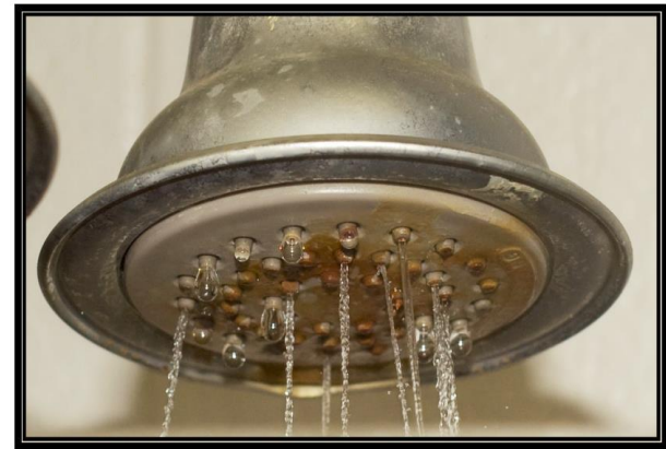
Figure 6-10D. Showerhead 10 on seventh day of testing with hard well water (28 grains per gallon) showing spray pattern. Battelle testing for Water Quality Association. May 1, 2009
