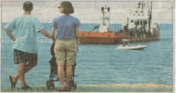
JUST ADD SAND: Beachgoers watch as the dredge Port Frederick begins depositing sand on Noosa's Main Beach.
