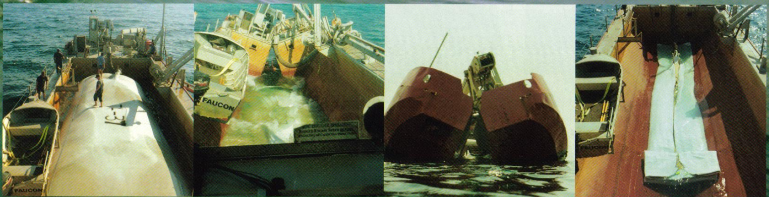
Above: Giant geotextile bags filled with sand ready to be placed on the sea bed
